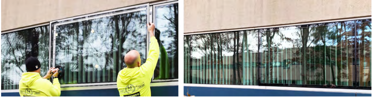
Exterior IGR retrofit of double-glazed windows, transforming them into triple-glazed without replacement.
